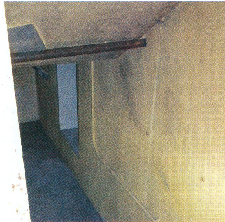
The entrance to a fallout shelter is down a flight of steps beyond a concrete door in the basement wall. A pipe, retrofitted after the end of the Cold War, holds the concrete door permanently open.
